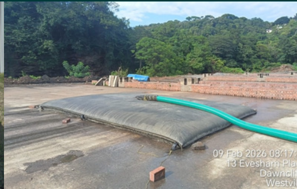
Titan tube demo unit after dewatering cycle of 2 days ready for more cycles
